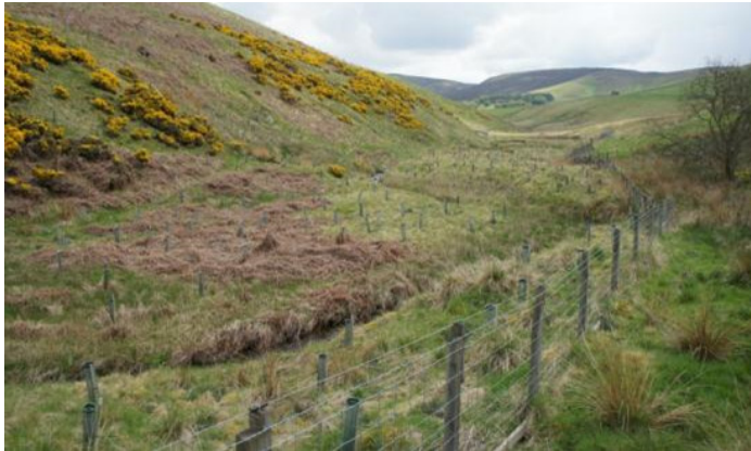
The picture on the left shows the slumped bank Along the Glendy Burn.
